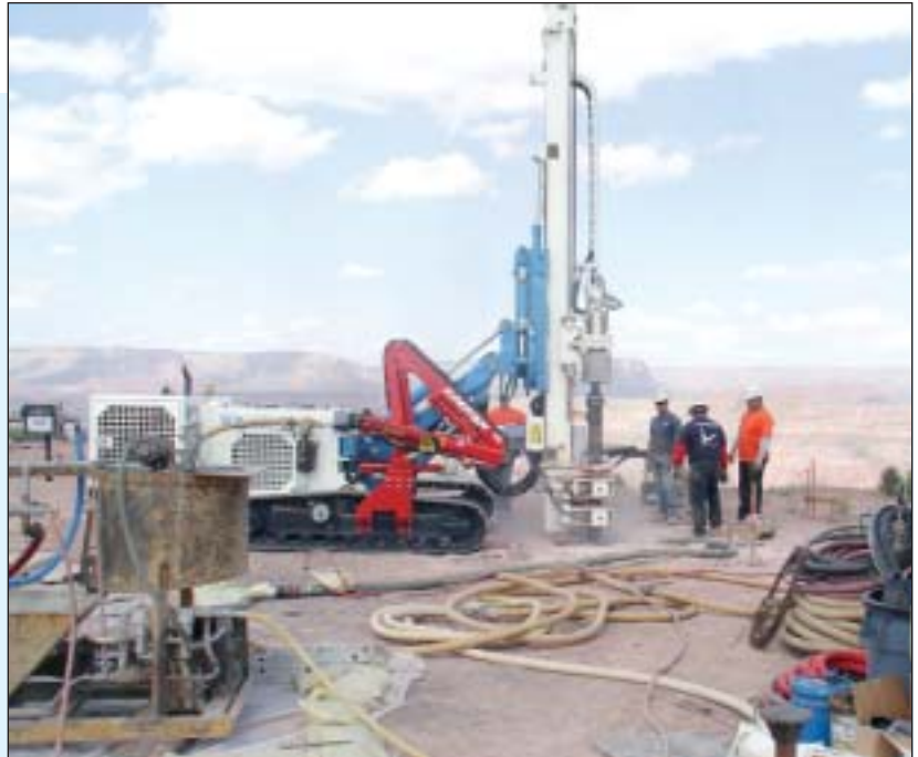
SoilMec 401 with down hole hammer drilling the perimeter of the pile cap.
