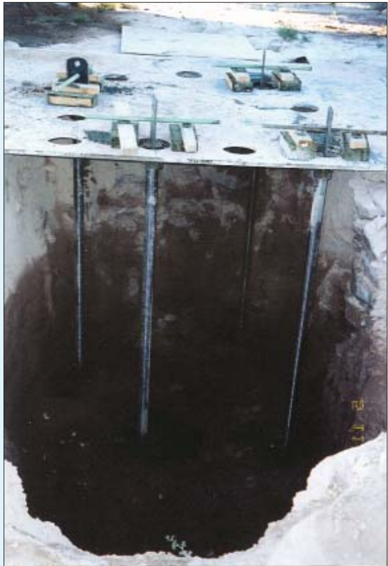
View of excavated pile cap with some of the vertical micropiles installed through steel plate template.
