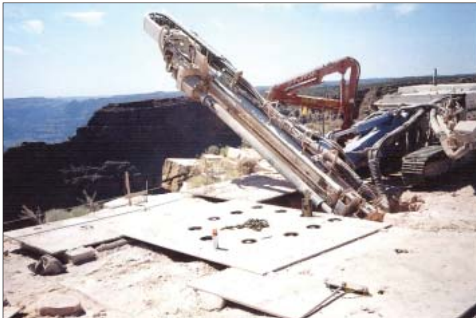
SoilMec 401 drilling one of three tiebacks for the pilecap plus the template for the micropiles.
